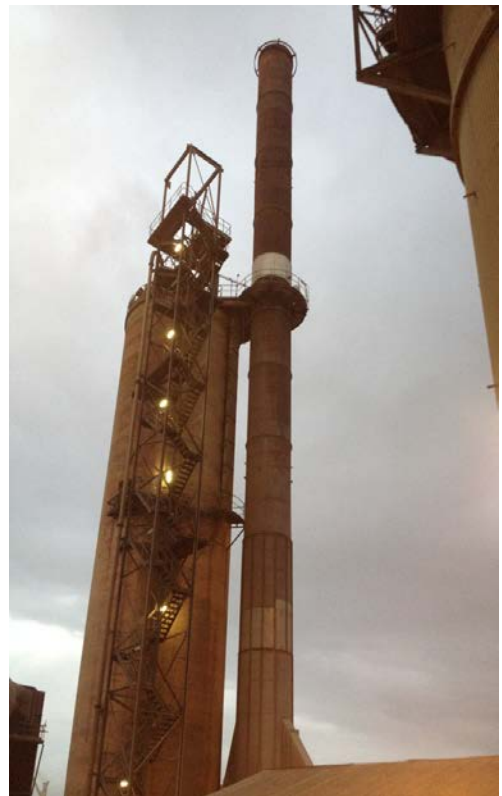
Figure 1: Kiln 4 Main Stack (RP 4A)
