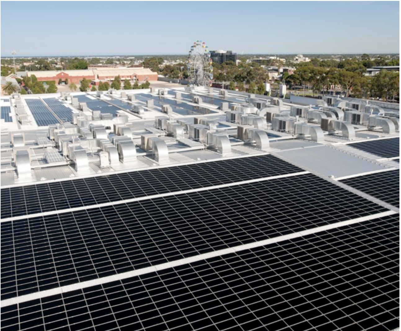
Solar installation, Adelaide Showground
